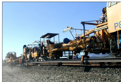
The P811 machine simultaneously dismantled and removed old track while placing new ties and threading new rail.
