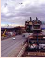
Airport MAX Red Line construction begins, as does construction of the Portland Streetcar.
